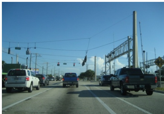
Strain-pole mounted signal at Copans Road
