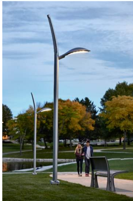
Signal Area and Pedestrian Lighting
